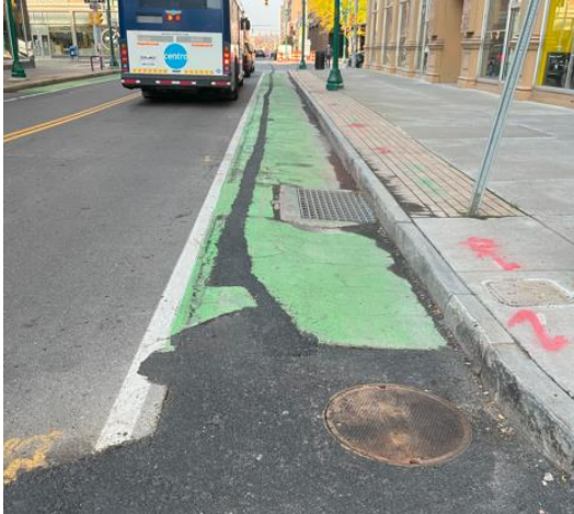
Contractors damaged this bike lane along E. Fayette Street
