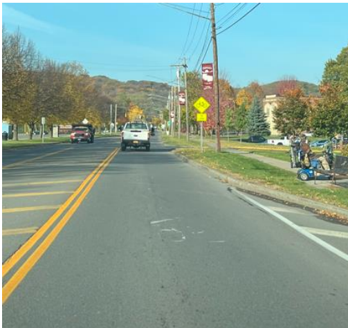
Badly worn out sharrows along W. Seneca Turnpike
