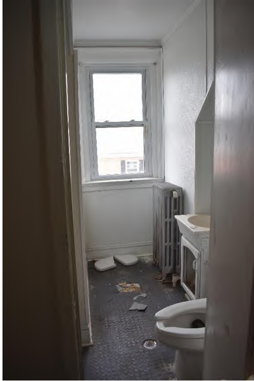
48. View of a bathroom. Note the vinyl wall coverings on the interior division.
