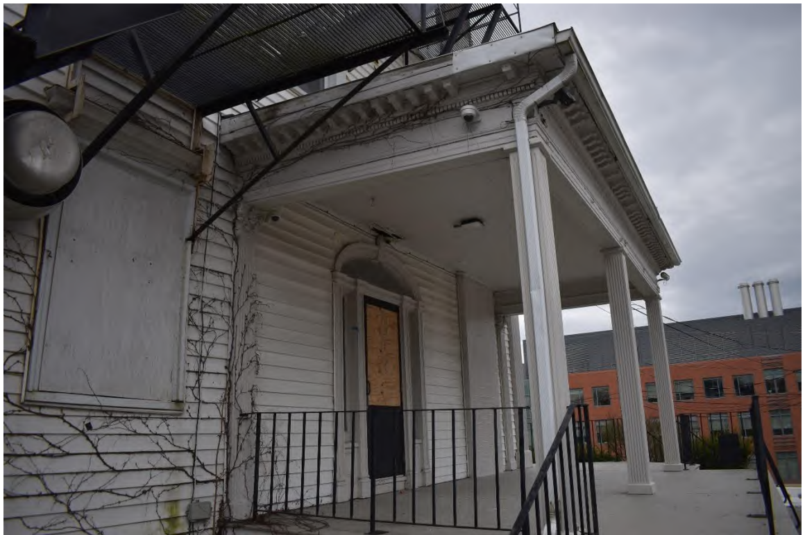
17. View to the southwest of the northern entrance. Note modern replacement materials throughout.
