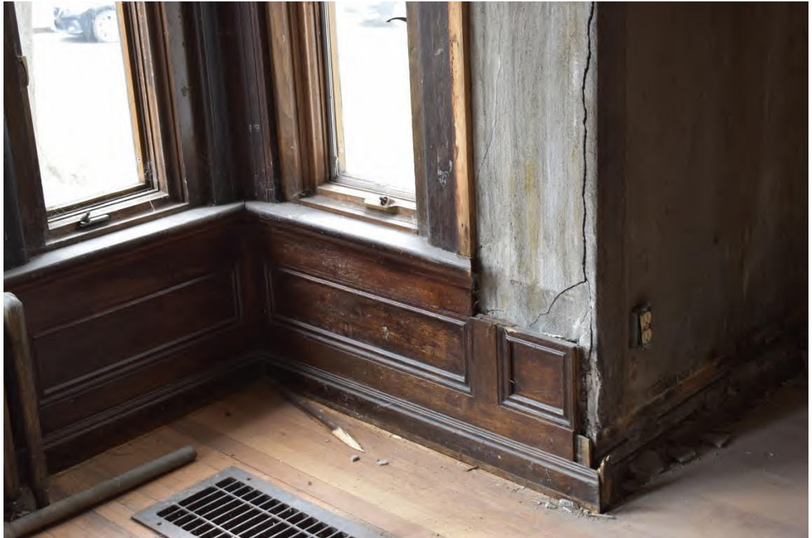
25. A small area of wood paneling remains underneath the casement windows in the box window.
