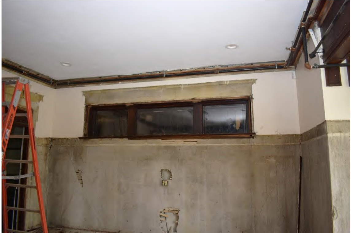
26. View of the leaded picture windows in the east wall of the dining room.
