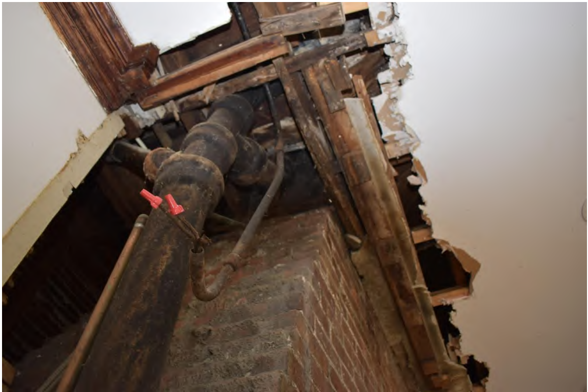
27. Evidence of water damage and structural repairs is evident in the exposed ceiling.
