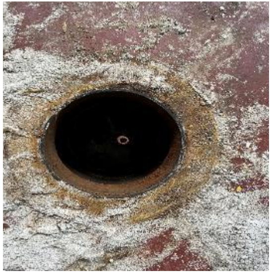
Photograph 14. In-hydraulic lift located inside the abandoned gas station.
