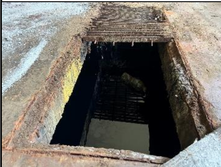
Photograph 11. Floor sump containing oil located inside the abandoned gas station.
