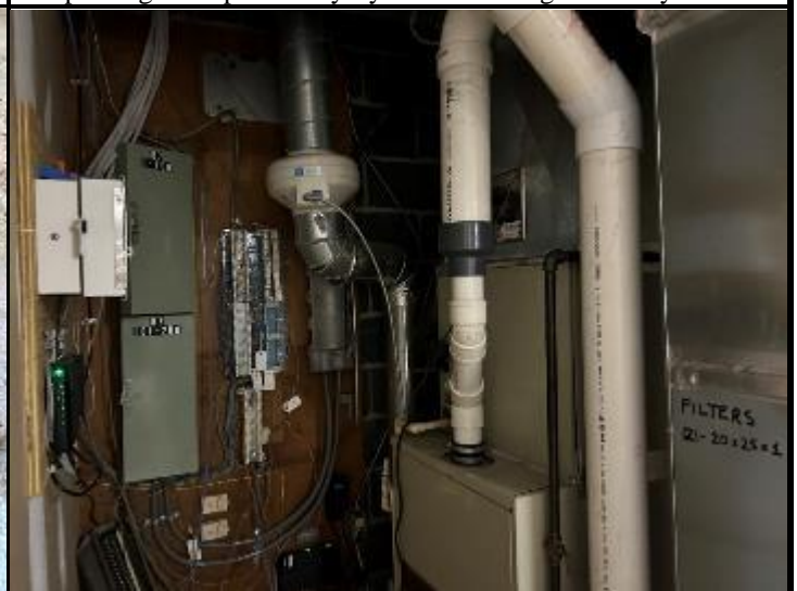
Photograph 12. Natural gas powered forced air furnace, located inside the vacant office building.
