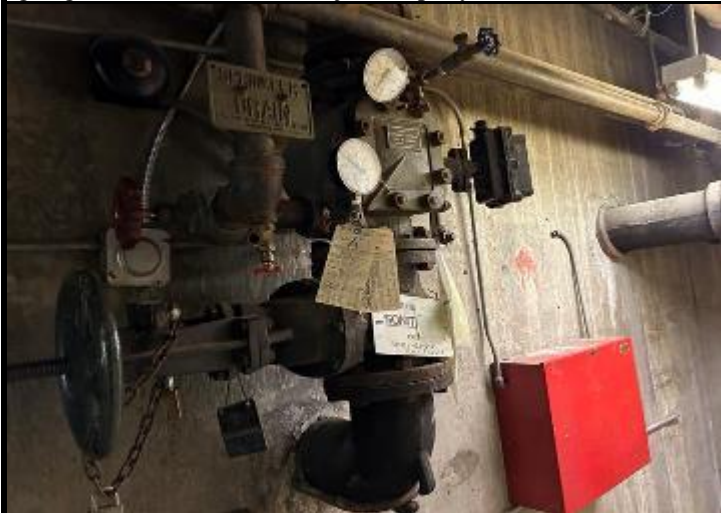
Photograph 5. Municipal water and sprinkler system located inside the vacant office building.
