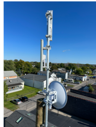
Utility Pole Mounted
